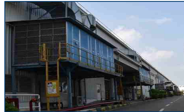
Air Handling Units at Site
