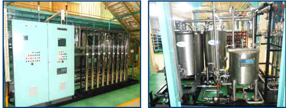
Electro Deposition Reverse Osmosis System
