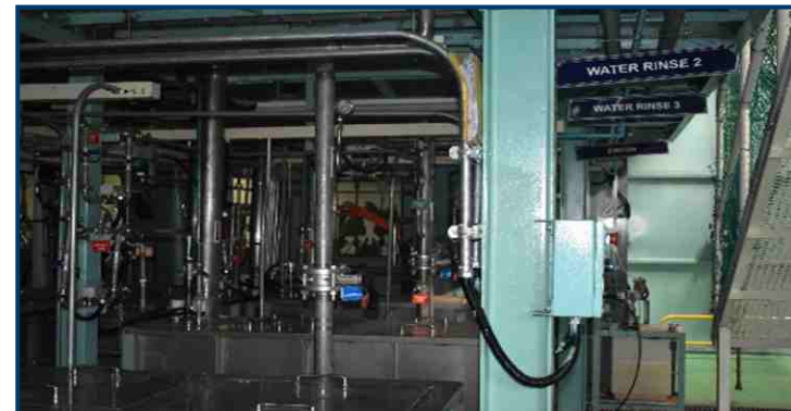
Electro Deposition Reverse Osmosis System
