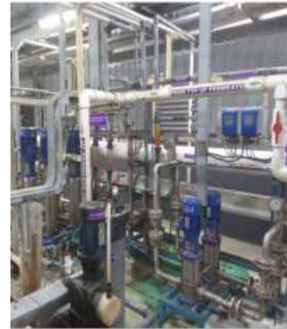
Fourth stage RO system is provided to recycle the effluent/ sewage further up to 97% and achieve the feed TDS of 40000 PPM to operate MEE effectively
