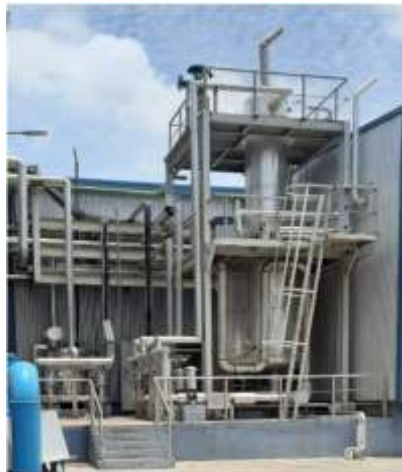
Spray chamber installed to recover the heat and water from venting steam
