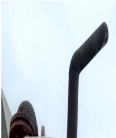
Process steam condensate main drain Flash steam venting to atmosphere
