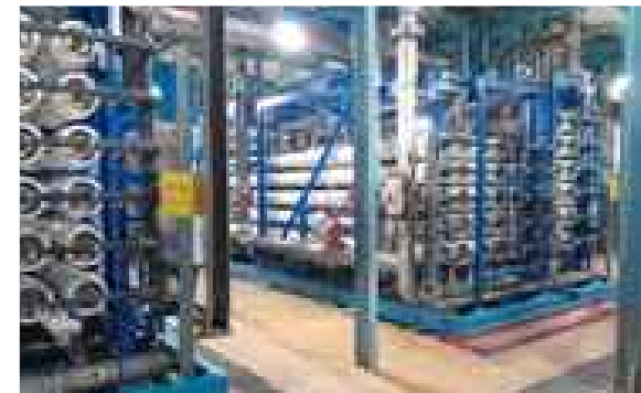
RO installed on treated effluent and other process streams
