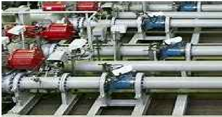
Flowmeters for consumption monitoring
