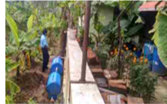
Grey Water Treatment Unit (WIP) at Chullimada Hamlet
