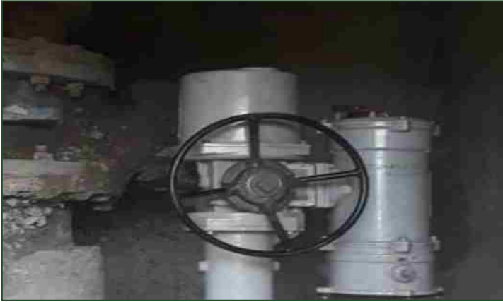
Fig. 8: BFV & Actuator for Controlling Application
