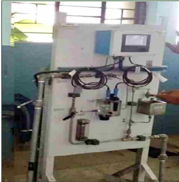
Fig. 10: PH/CL/Turbidity Analyzer Panel
