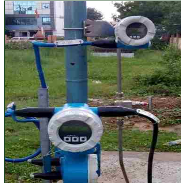
Fig. 11: Flow meter & Pressure Monitoring Device installation
